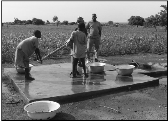
Concerned Christians make it possible for Ganaians to have deep bore wells.
